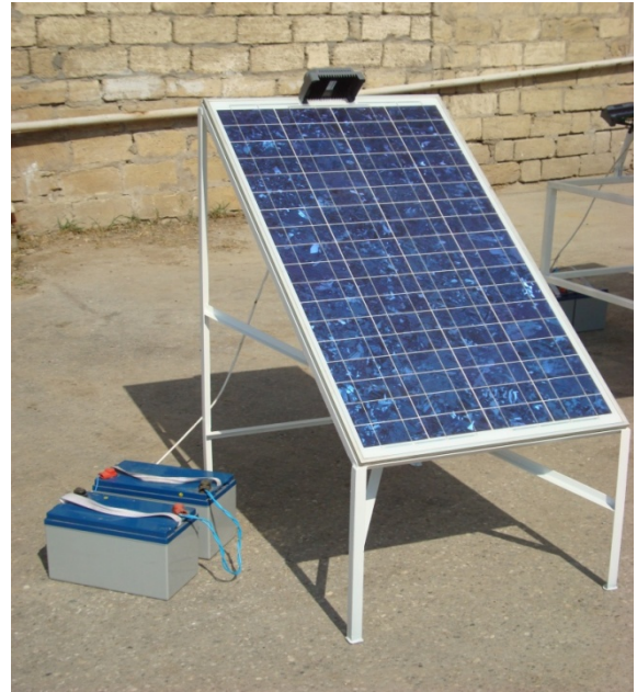
Picture 1. Solar PVs, controller and accumulator
