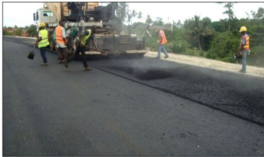
Figure 6. Correcting segregation by broadcasting HMA on defective areas
