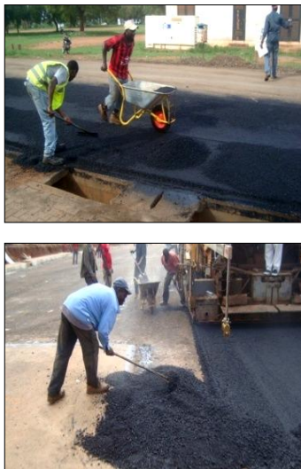
Figure 2. Improper manual placement of HMA
